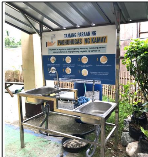
Figure 2. Portable Handwashing Facility from Plan International
